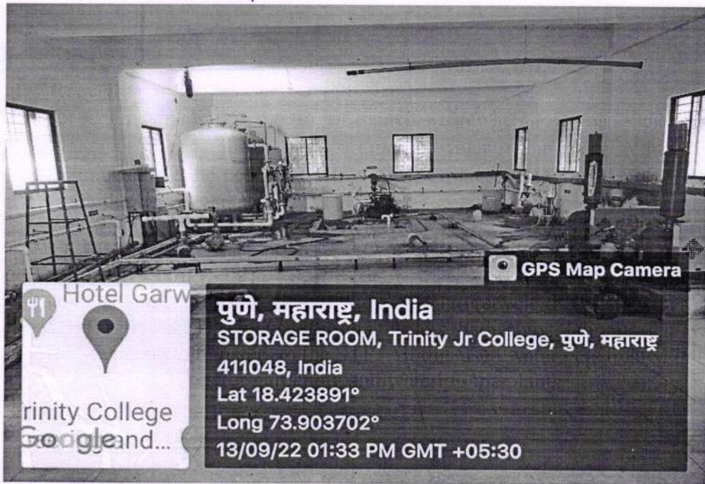
Sewage Treatment Plant (STP)
