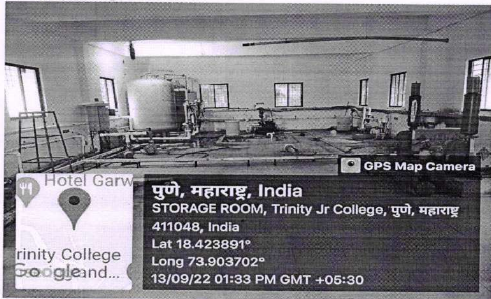
Sewage Treatment Plant (STP)
