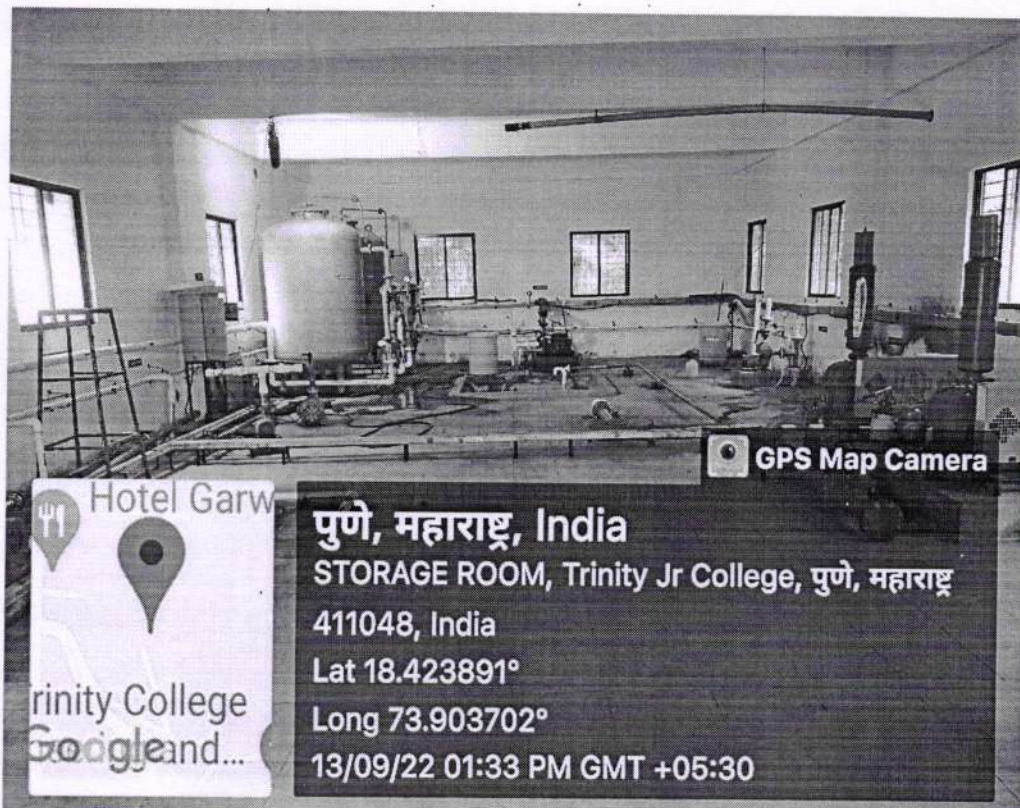
Inside view of STP
