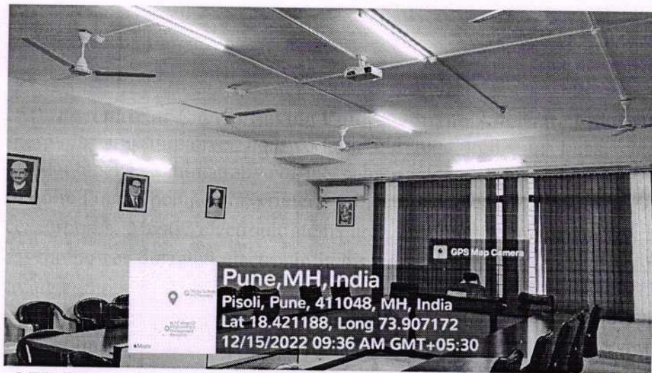
LED lights and energy saving equipment (Projector and AC) in board room
